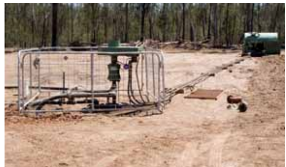
Typical coal seam gas production well. Photo courtesy of Arrow Energy Limited
